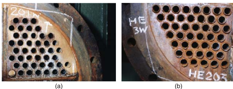
Case 35 (a) Inlet end erosion corrosion of carbon steel tubes in an acid cooler, first pass. (b) Inlet end erosion corrosion of carbon steel tubes in an acid cooler, second pass.
