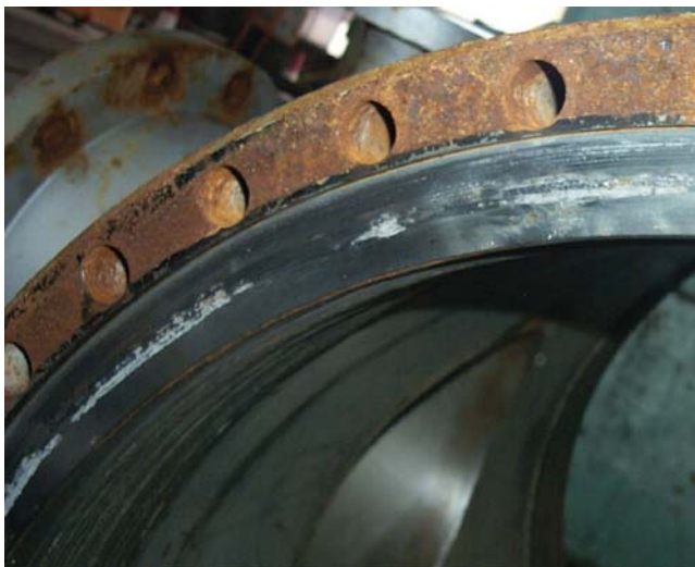
Figure 3.6 Photograph of a part of heat-exchanger sheet affected by crevice corrosion. The carbon steel shell was weld-cladded with SAF 2507 alloy. Note, only the gasket area of the shell suffered from attack; shell side was exposed to seawater. (Source: Raja (2008). Reproduced with permission of Narosa Publishing House.)
