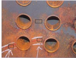
Case 17 Cracks on mud drum shell in a coal fired steam boiler.
